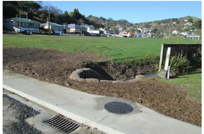
The new inlet structure at the Ward Street open space. The open storm water drain accepts water from Elizabeth Street and Hill Street.
