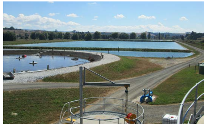
Te Kuiti Wastewater Treatment Plant.
